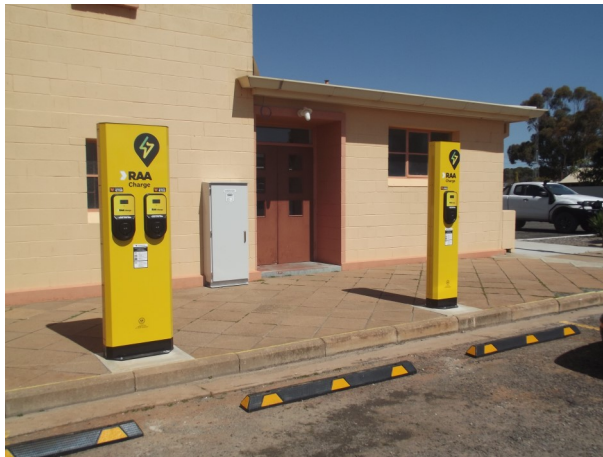
Part of the Electric Vehicle (EV) Charging Station adjacent to the Town Hall on Cross Street.
