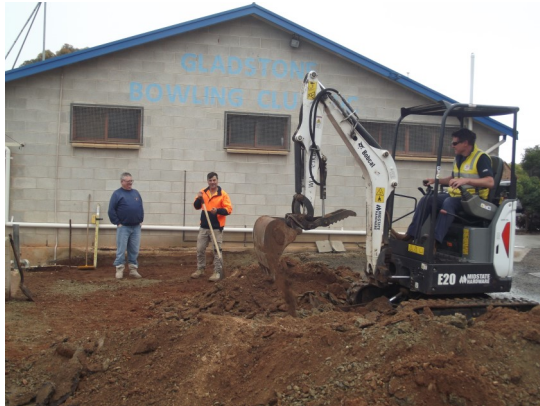
Graeme Smith and Tim Zander inspecting the site for the new sheltered area at the Bowling club. Luke Frost is operating the digger.
